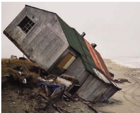
A Shishmaref home tumbled onto the beach after rising seas undermined the bluff where it sat.
